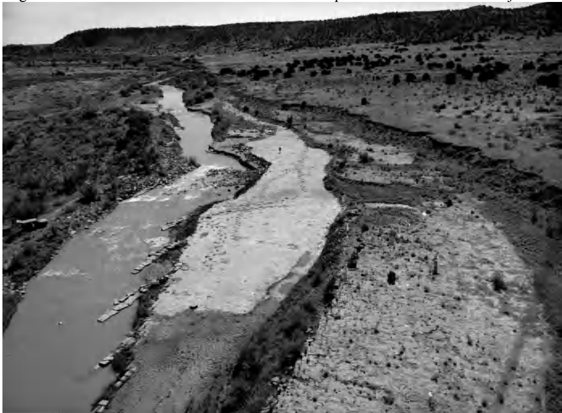
Picketwire Canyonlands, SE Colorado - Rock vanes used to protect dinosaur trackway. These structures were installed in 1998, and survived a 100 year event the following spring. Note the deposition and new willow vegetation taking hold in between the structures.
